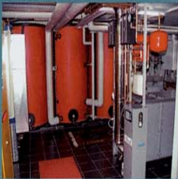
buffer storage tanks
