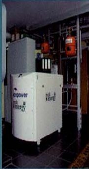
CHPU: providing thermal and electric energy
